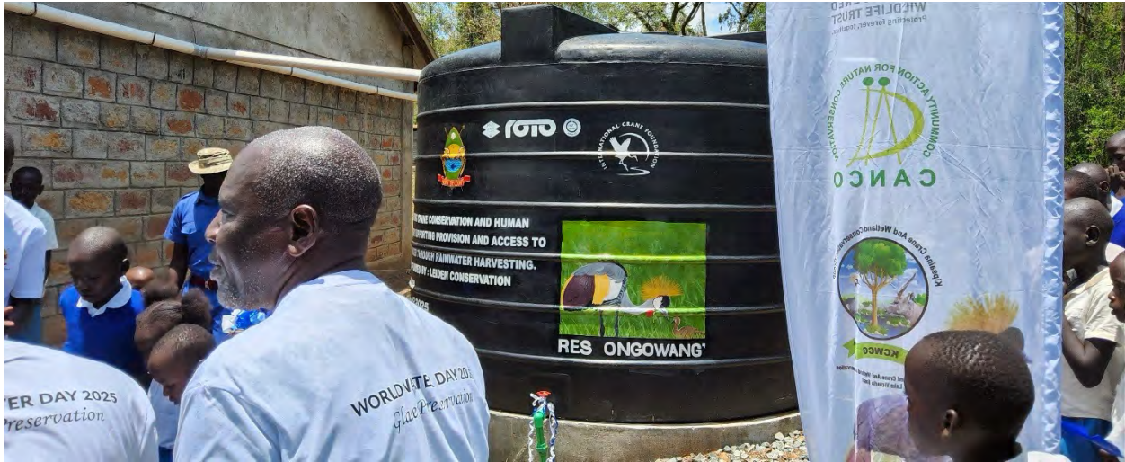
Image 8: Water tank installed at Kisamba Comprehensive School in Homa Bay County.
