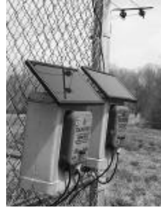
Fig. 11F.2. Electric fence and solar charge units.
