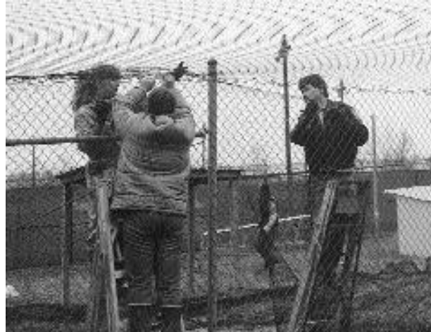
Fig. 12.11. Nets are attached for easy release by hooking the mesh over the cut-ends of the chain link fabric. Photo George F. Gee
