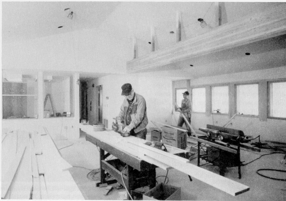
ICF's General Contractor, Ken Decker, put finishing touches on the reading room of the Ron Sauey Memorial Library for Bird Conservation. Serving ICF staff and conservationists from this country and overseas, the library will house collections on ornithology and conservation, and provide wider access to scientific literature through a computer network. ICF is seeking donations of books to the library. Photo by D. Thompson.
