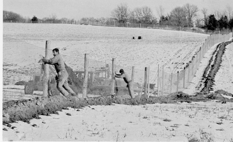
As a first step in the construction, the entire perimeter fence went up this fall. It will keep predators and unauthorized people away from the breeding cranes.
